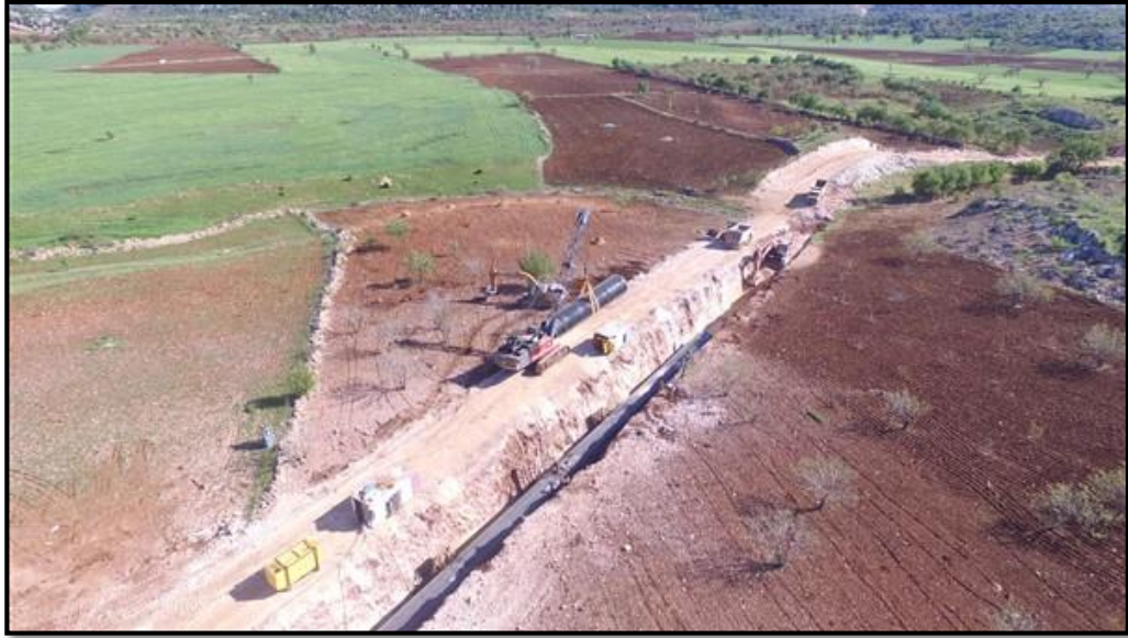
Figure 5.3 Transmission line of Düzbağ Dam
