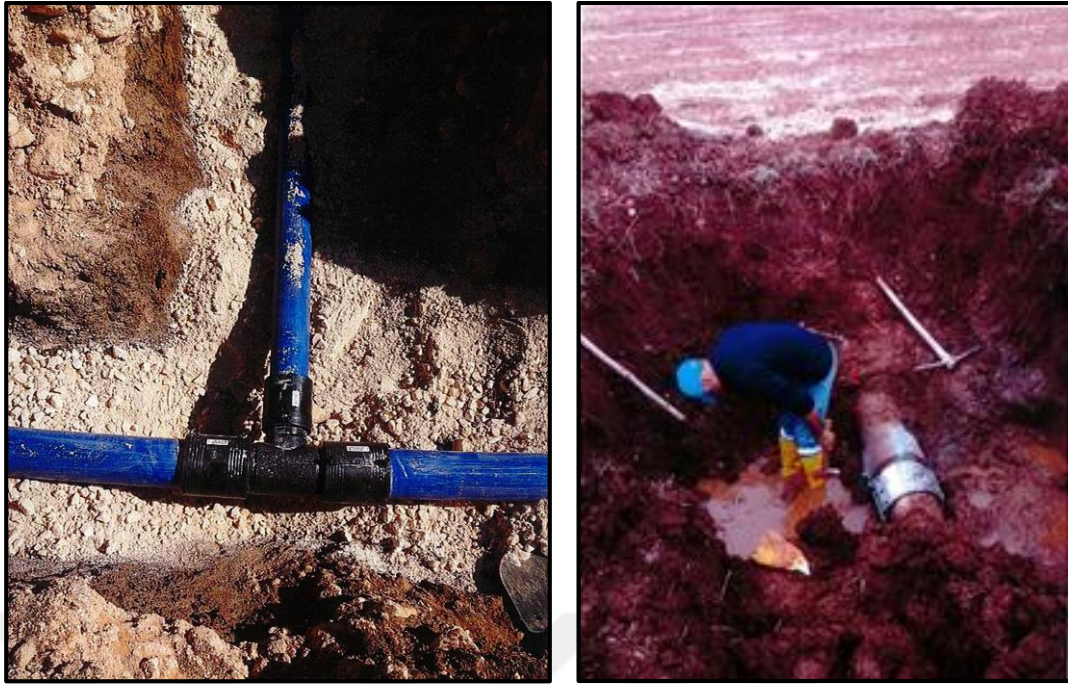
Figure 4.2. Example of Leakage Management
