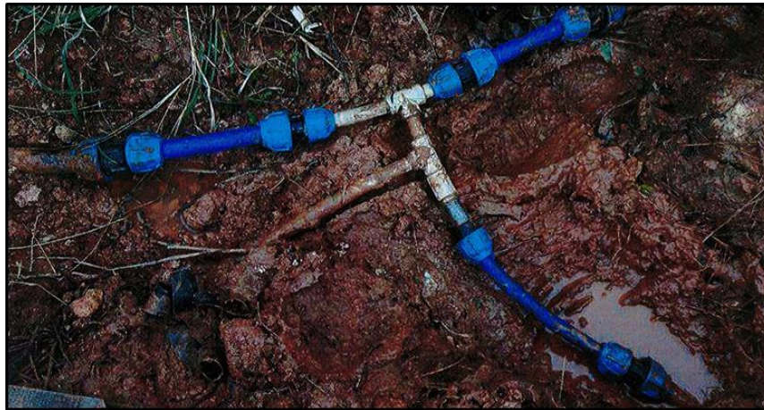
Figure 3.6. Example of Incorrect Fitting (Physical Water Losses)
