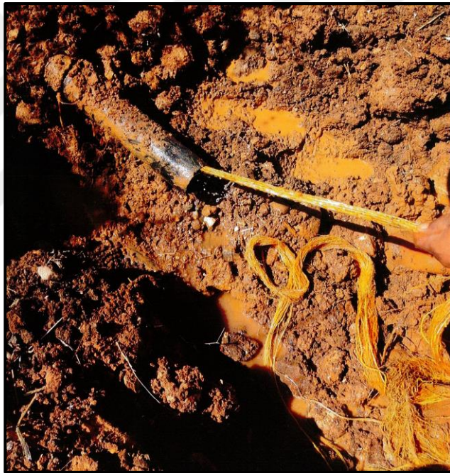
Figure 3.2.Example of Poor workmanship in fittings (Physical Water Losses)
