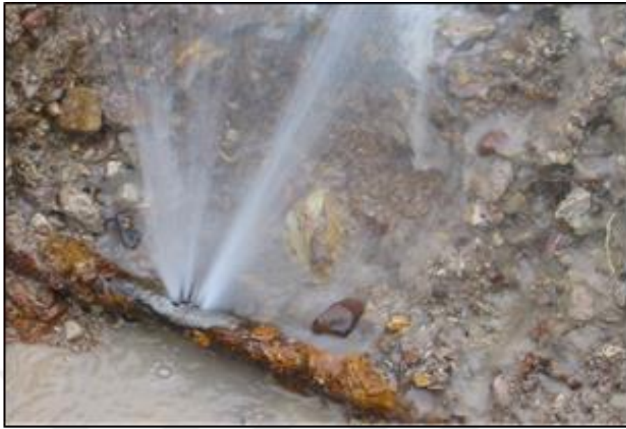
Figure 3.3.Example of Aging and Corrosion of the Pipe (Physical Water Losses)
