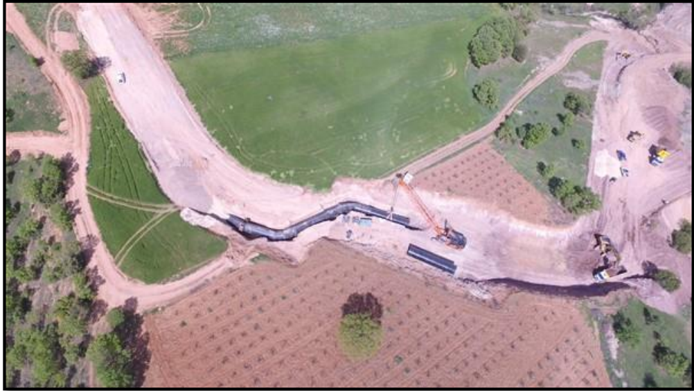
Figure 5.1 Transmission pipeline of Düzbağ Dam
