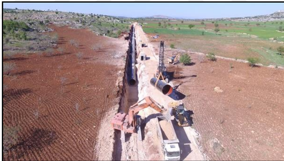
Figure 5.2 Transmission line of Düzbağ Dam
