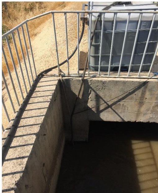
Figure 3.7 Taking wastewater from the influent water of the plant to the first sedimentation tank by pump.
