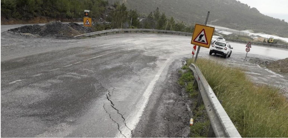
Figure 3.6. Cracks on the D400 highway above the T-8 tunnel.
