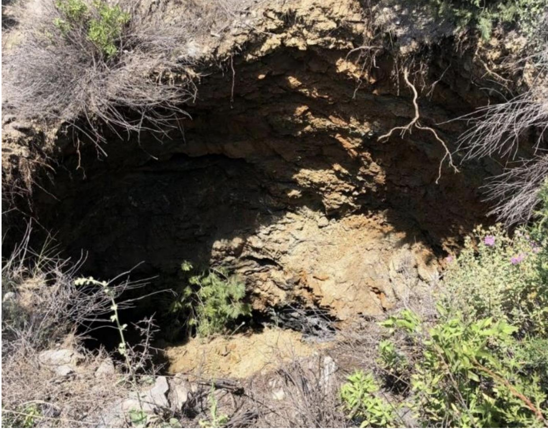
Figure 3.7. Surface of the sinkhole that is occurred in the T-8 north tunnel.
