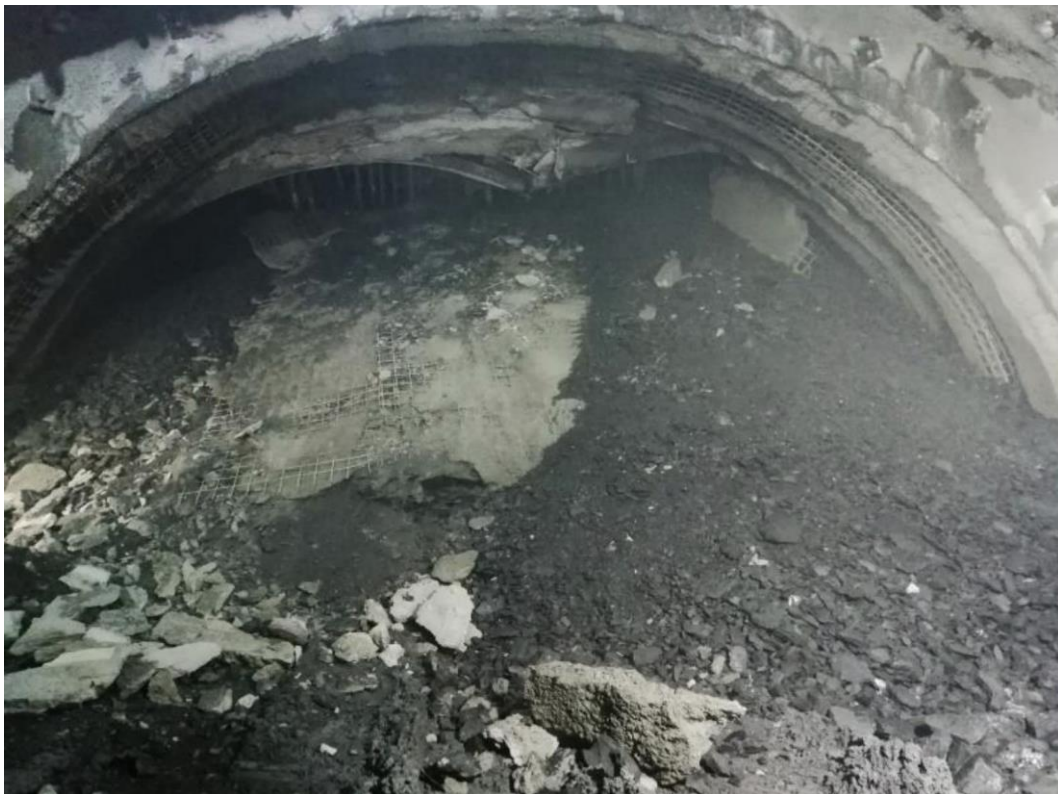
Figure 3.5. Photo of deformation and collapse in the T-8 north tube.
