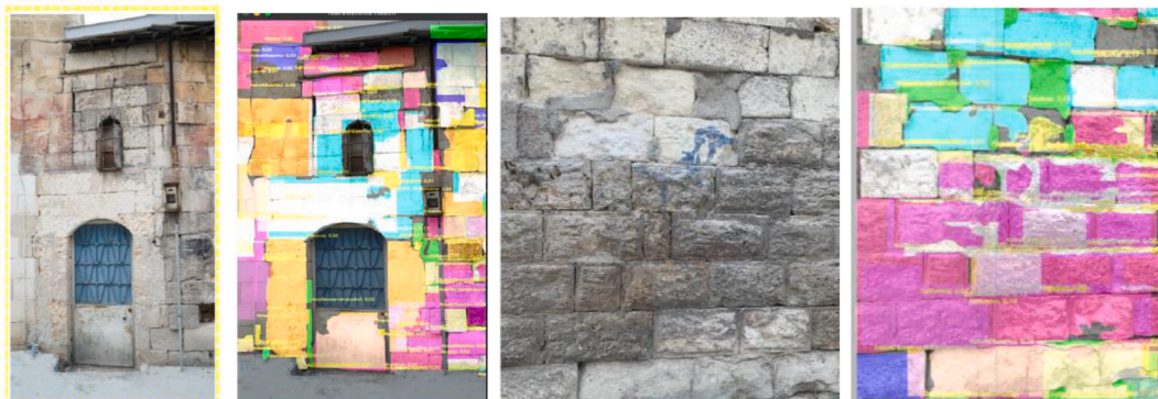
Fig. 9 677 Block 46. Parcel street frontage image and artificial intelligence-supported deterioration map estimation.
