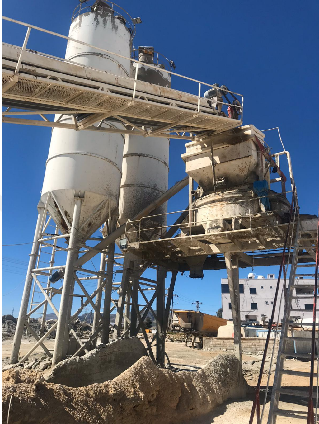
Figure 2.7. Ready-Mixed Concrete Plant
