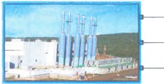
Diesel Generator 15 MW (Source)
