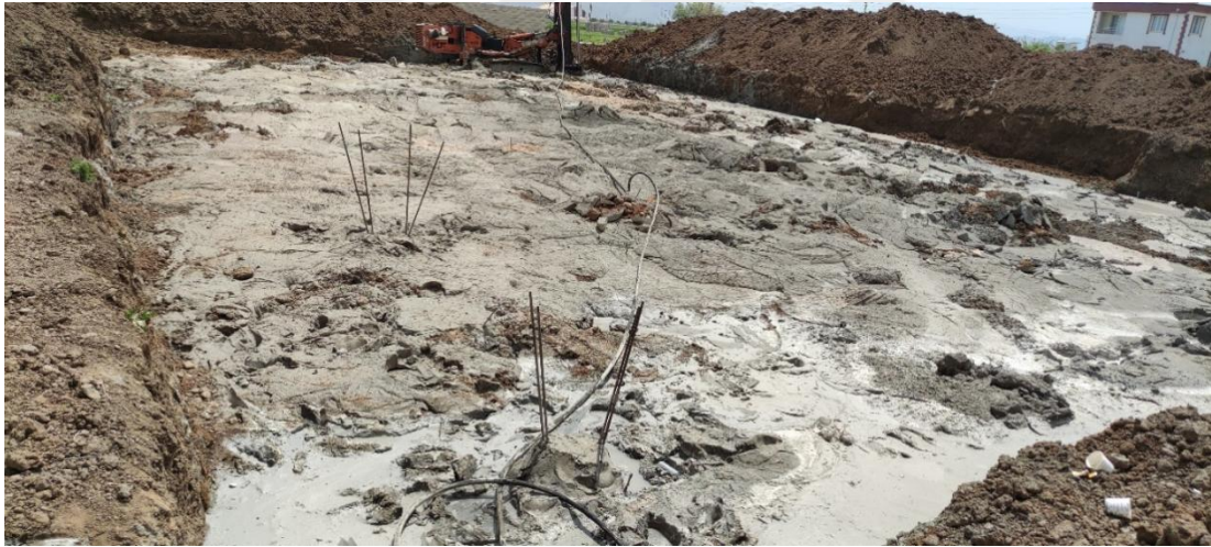
Figure 2.12 An image of the Jet Grout work performed in the study area.
