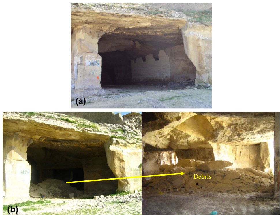
Fig. 6 General views of opening 5. a Before the collapse, b after the collapse
