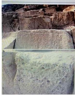
Figure 2.5. a, b Cracking and splitting of backing limestone blocks at Giza
